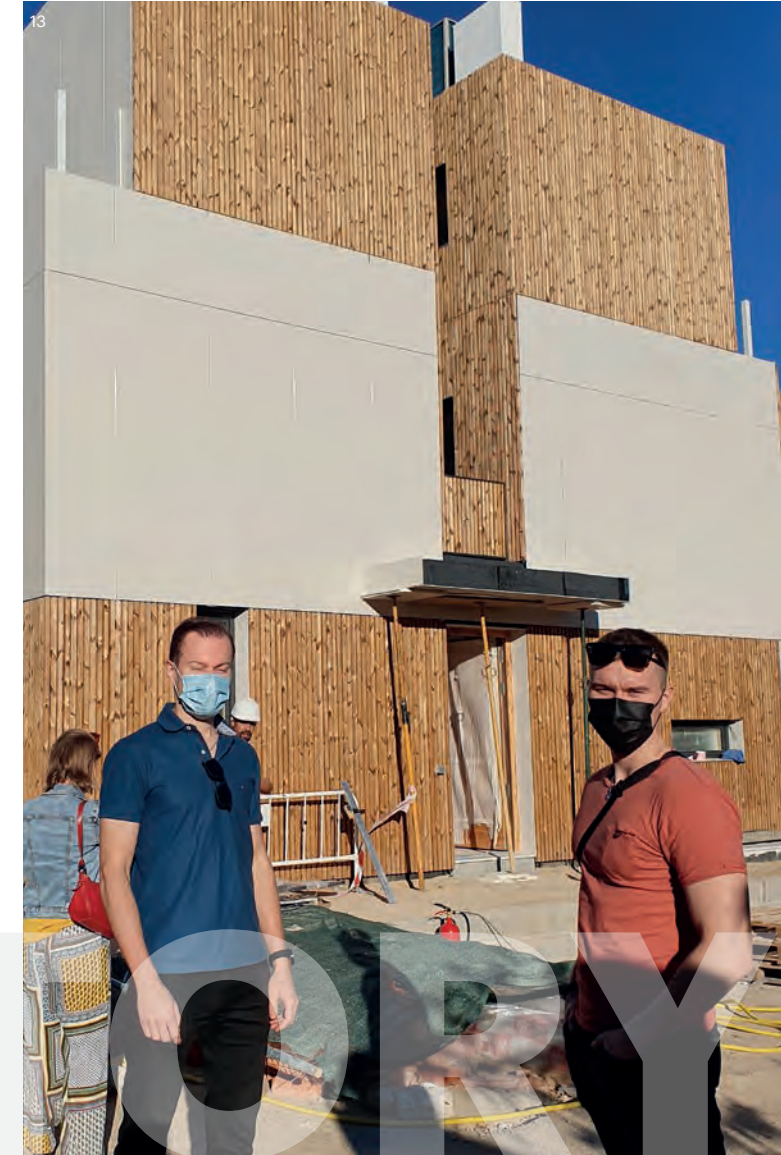
Lunawood ambassadors on the building site of a beautiful private home in Madrid.
